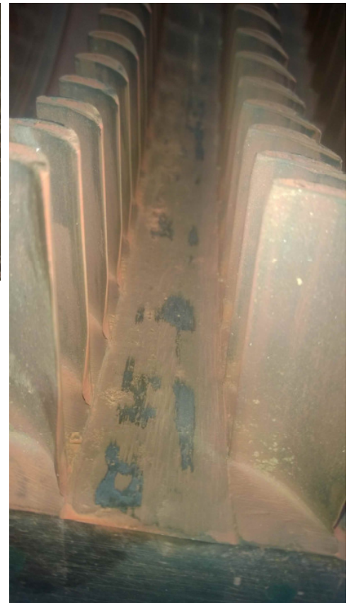
Lower HP casing - Left side
