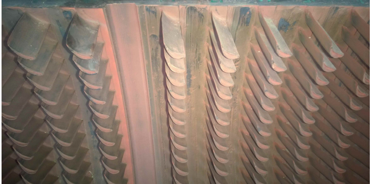
Lower HP casing - Left side
